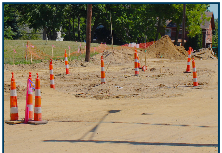
A new roundabout is under construction at the intersection of MLK Drive and Morrell Street.
