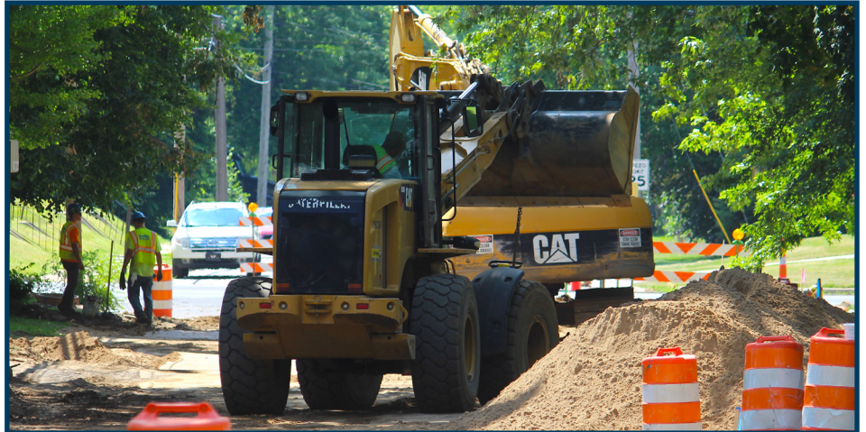
W. Franklin Street is under construction from S. Brown Street to S. West Avenue.
