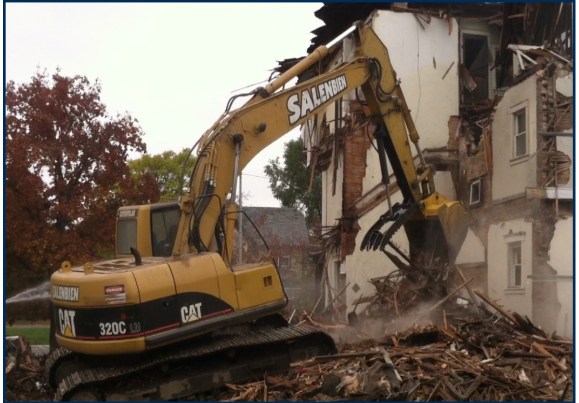
A contractor demolishes a structure within the City of Jackson. A new report shows that the demolition program has saved millions in home value.
