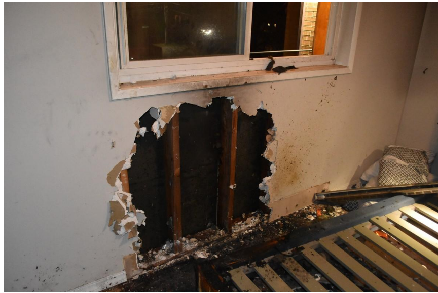
Fire caused by items too close to baseboard heater
