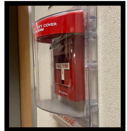
Covered alarm pull station
