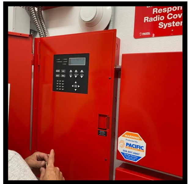
Fire alarm panel
