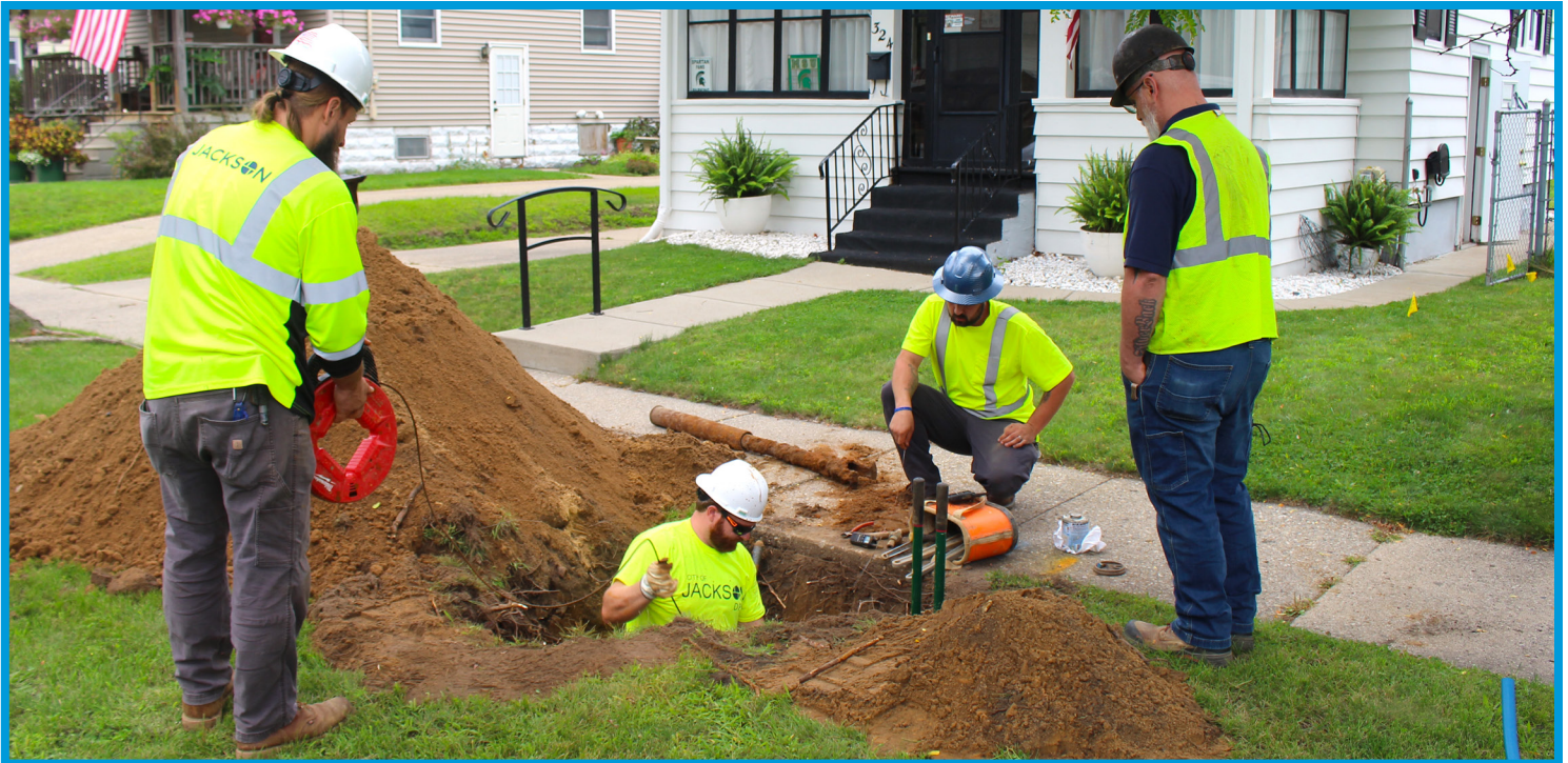
Lead service line replacement crew from DPW replaces service line at a home on Bates Street in Aug.
