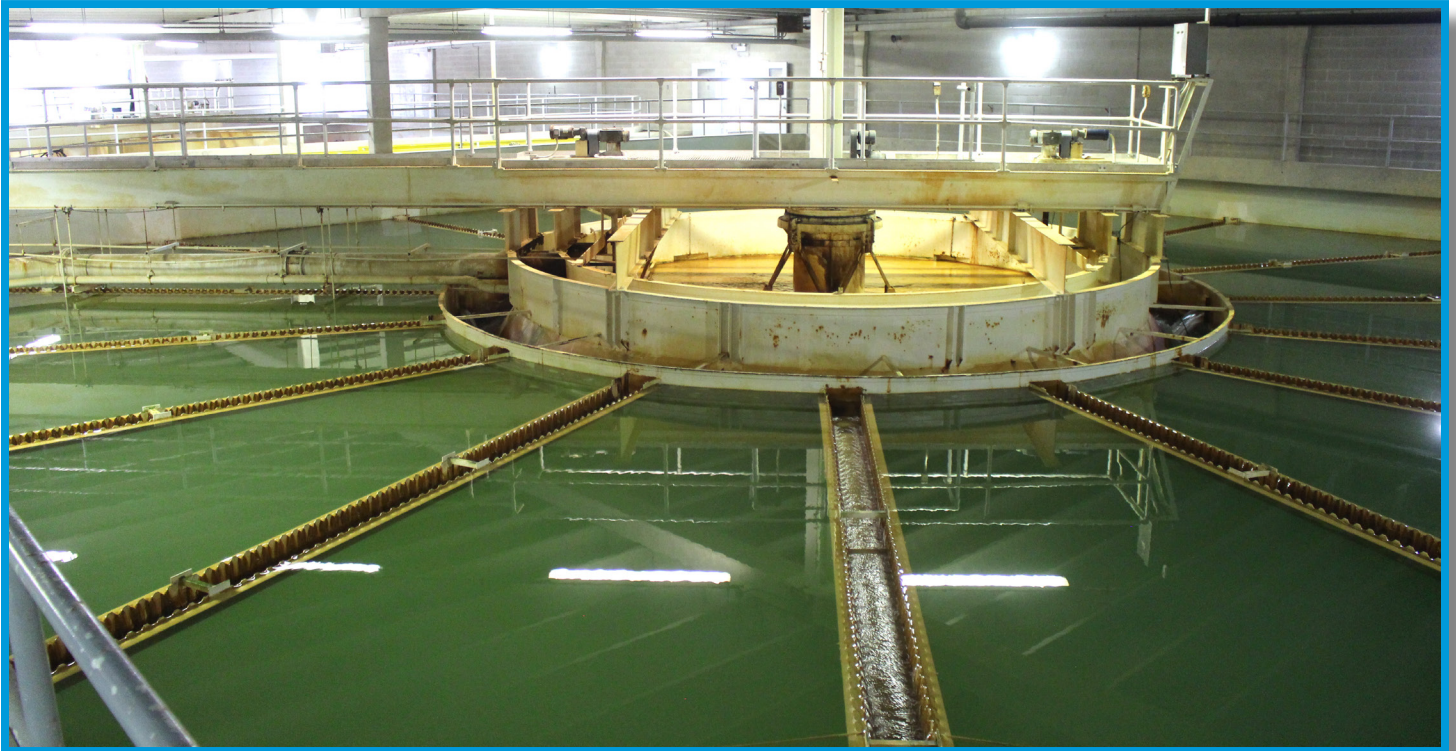
Photos of the City of Jackson Water Treatment Plant.
