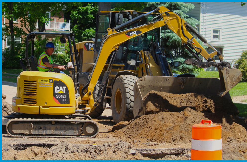
Water main and lead service line replacement project on S. West Ave.
