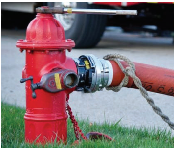
Storz fitting on a hydrant
