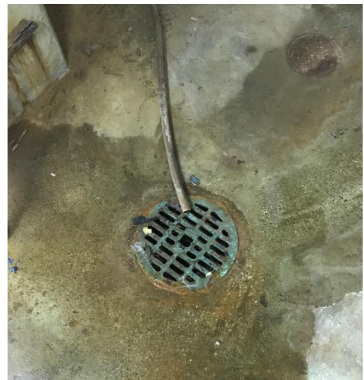
Figure 3-4 - Floor drains are showing signs of corrosion.
