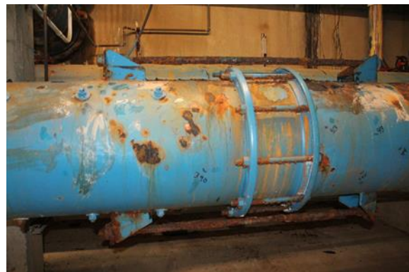
Figure 4-6 - Example of severely corroded mechanical coupling hardware.
