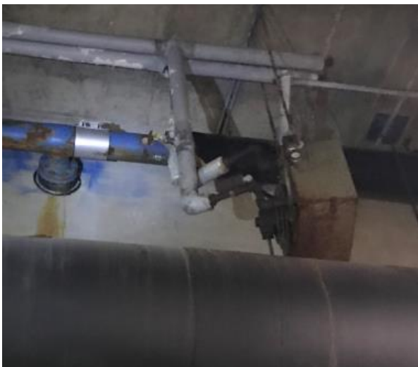
Figure 5-8 - Unit Heater ineffective since the new dehumidifier will have heating.
