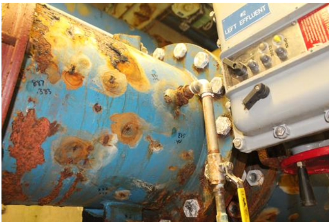
Figure 4-5 - Severely pitted surface with unknown thickness due to limitations of the UT instrument.
