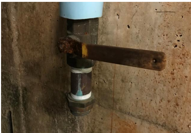
Figure 3-3 - Service water drain valve handle showing signs of corrosion.
