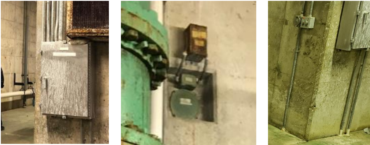
Figure 5-6 - Corrosion in junction boxes.
