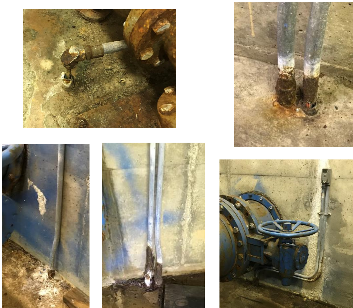
Figure 5-1 – Cables fully exposed from a corroded conduit.
