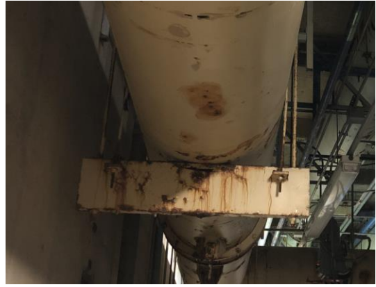
Figure 6-1 - Typical large diameter pipe support.
