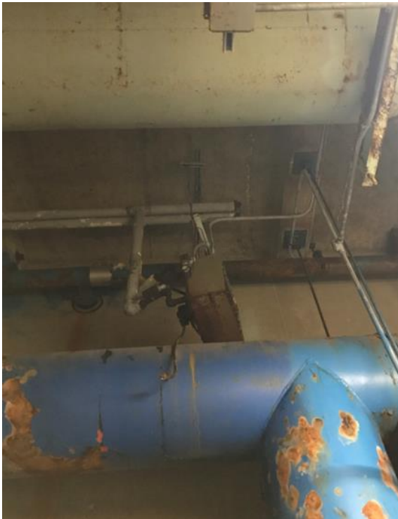
Figure 3-1 – Unit heaters serving piping gallery are beyond their useful life, corroded and are not operational. Heat will also be provided by new dehumidification unit.
