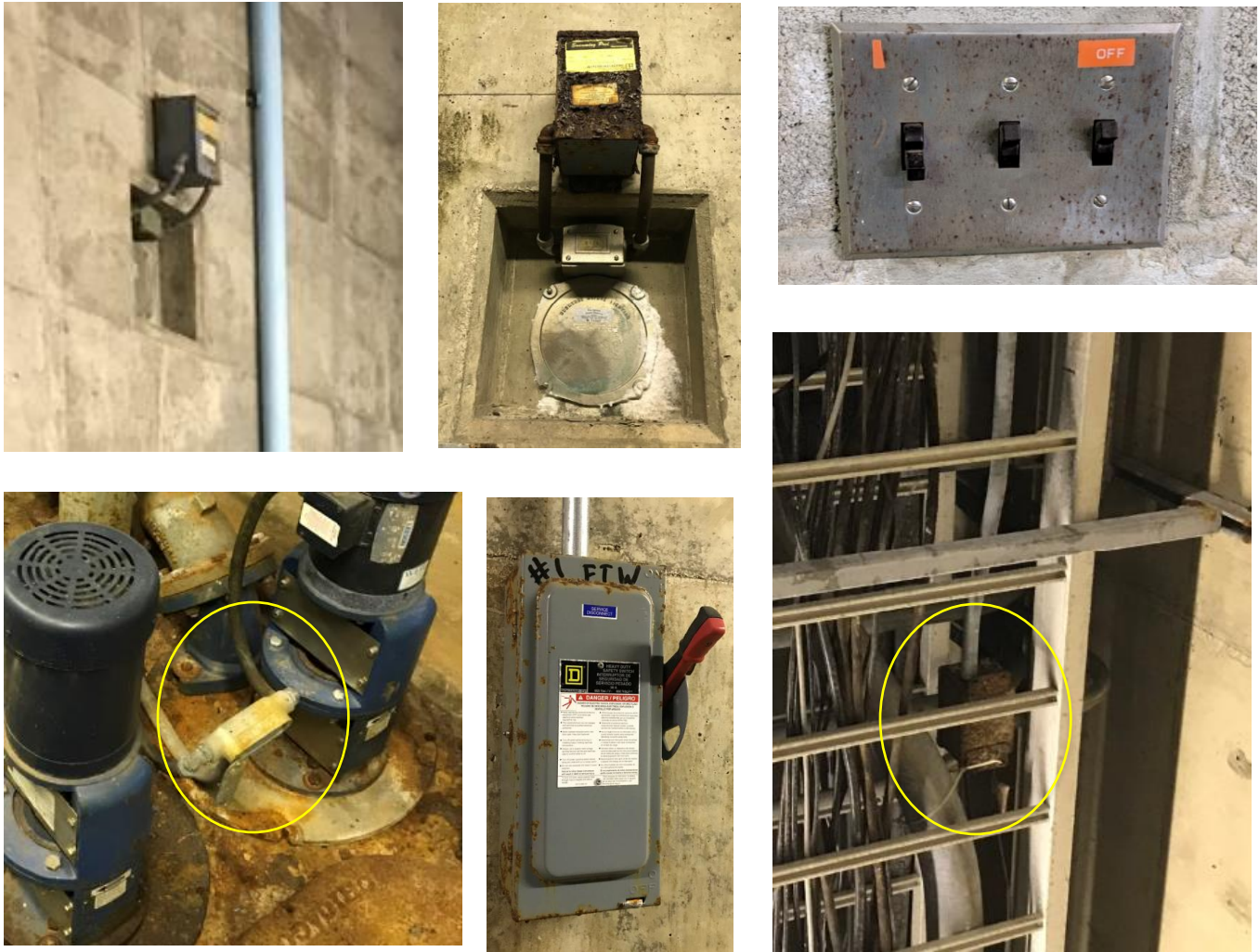
Figure 5-7 - Corrosion in various electrical devices.
