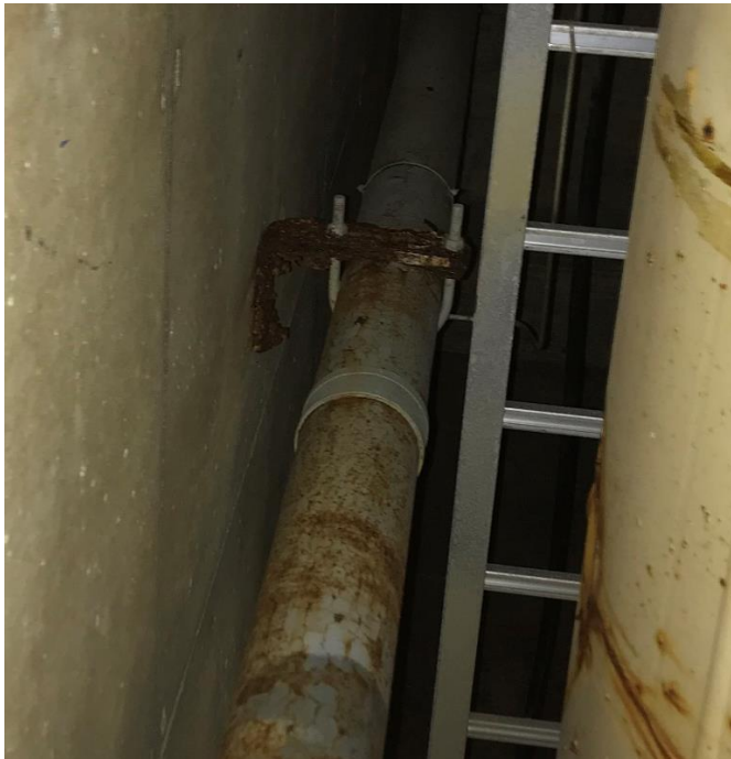
Figure 3-5 - Vent/sanitary waste piping wall supports are showing signs of corrosion. Vent/sanitary piping showing signs of corrosion.
