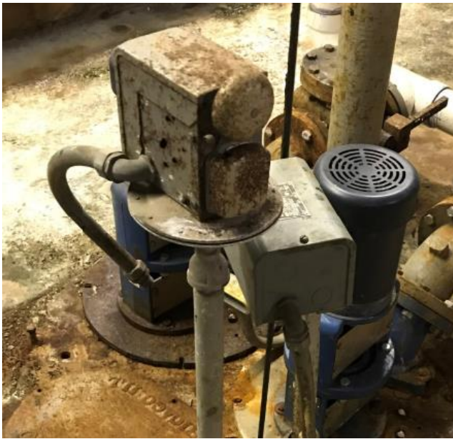
Figure 5-9 - Sump pump motor corrosion.
