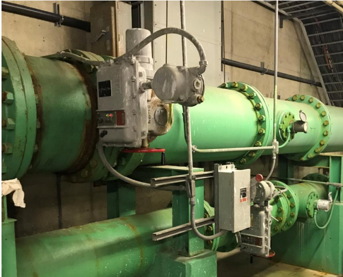
Figure 5-2 - Paint streaks and rust on an actuator and gear box.
