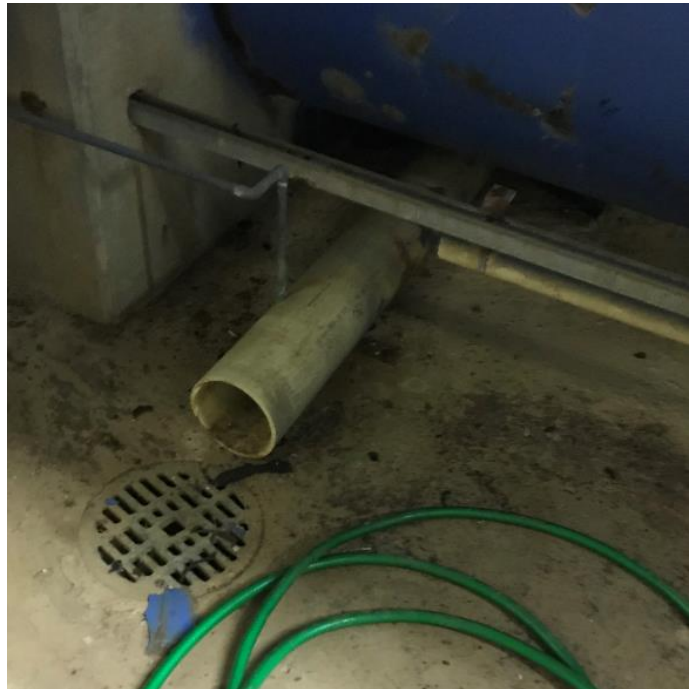
Figure 3-6 - Sink drain does not align with floor drain, causing unnecessary puddles on floor.
