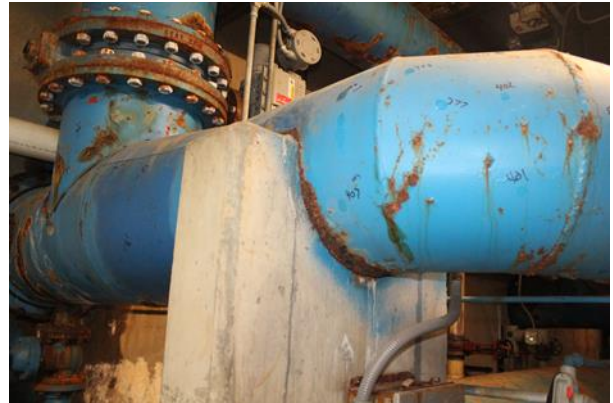
Figure 4-2 - Example of corrosion at pipe supports.
