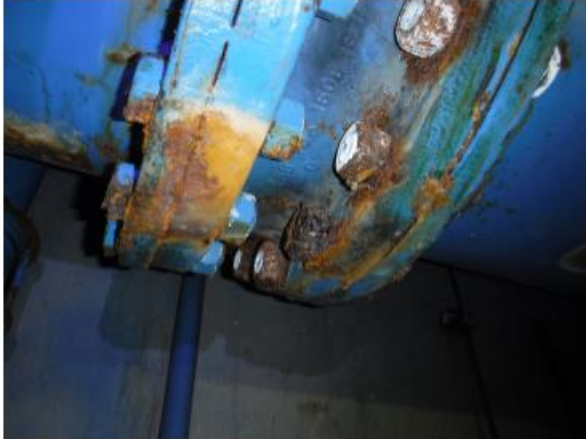
Figure 4-7 - Example of severely corroded flange hardware.
