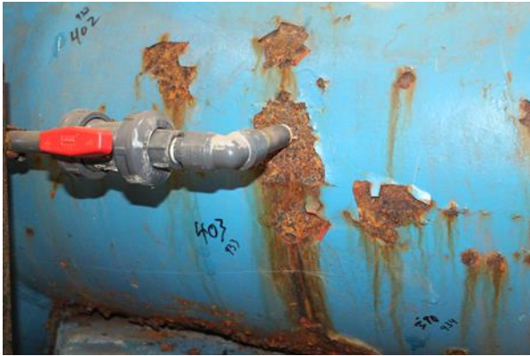
Figure 4-1 - Example of corrosion at pipe taps.
