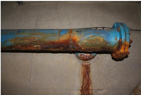
Figure 4-3 - Surface wash piping is severely corroded throughout the piping gallery.
