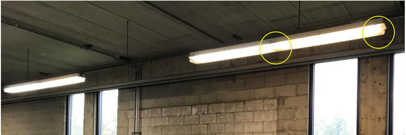
Figure 5-10 - Rust is visible in some of the general lighting frames.
