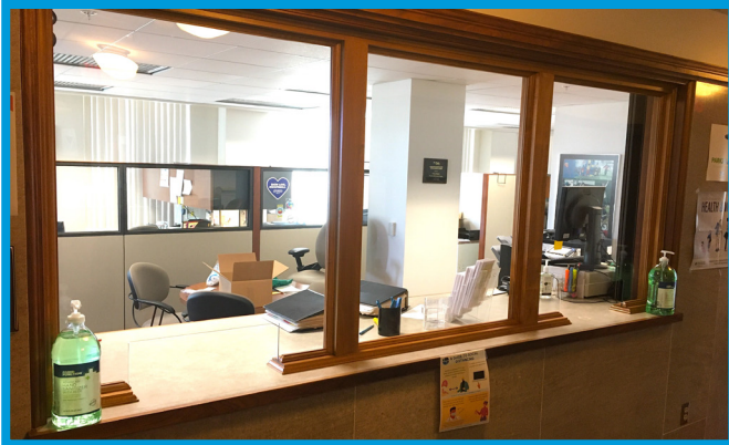
New service windows with protective glass were installed in every City department that interacts with residents in person.
